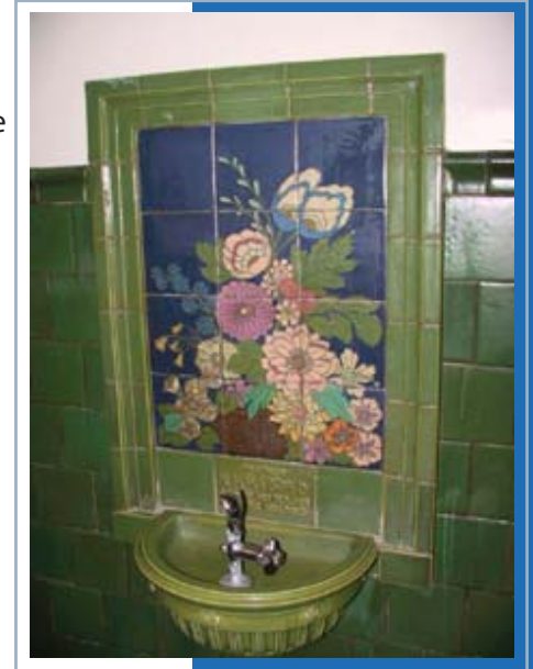
One of 24 rare Rookwood art tile drinking fountains found in Cincinnati Public School buildings.
